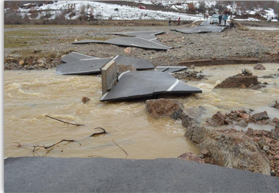
Road connecting Klina and Malisheve was disrupted 9 due to floods in January 2021
