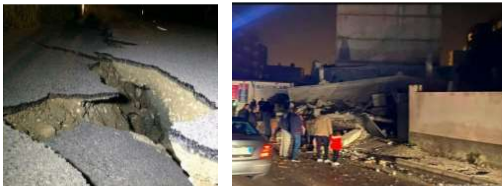
Figure 14: Damaged roads and other infrastructure in Albania after the earthquake, 2019
