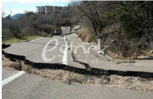
Figure 30: Landslide on the main road Cetinje Budva, 2015
