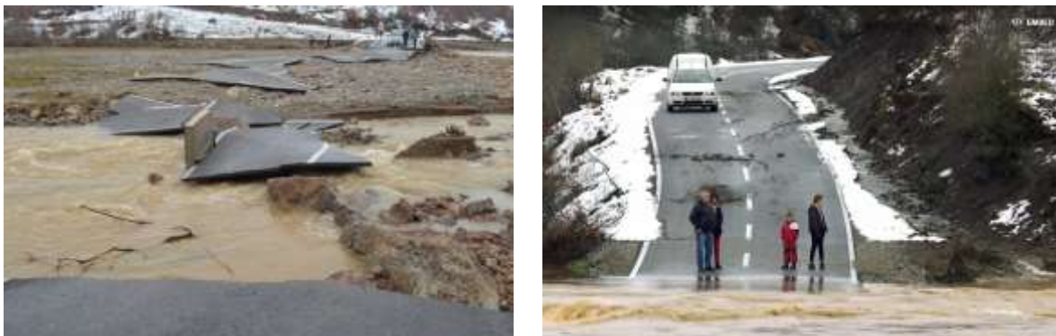
Figure 25: Road status after floods in 2021 13
